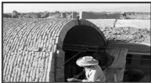
F6. Leveling the vault using ropes. Place of construction: Abarkouh, Yazd Province, vault restoration (Source: Negarandegan).
